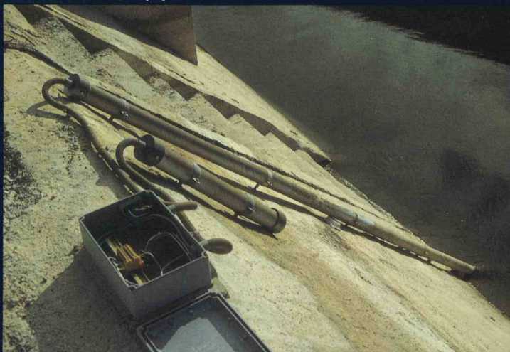
Canal level meter and alarm
