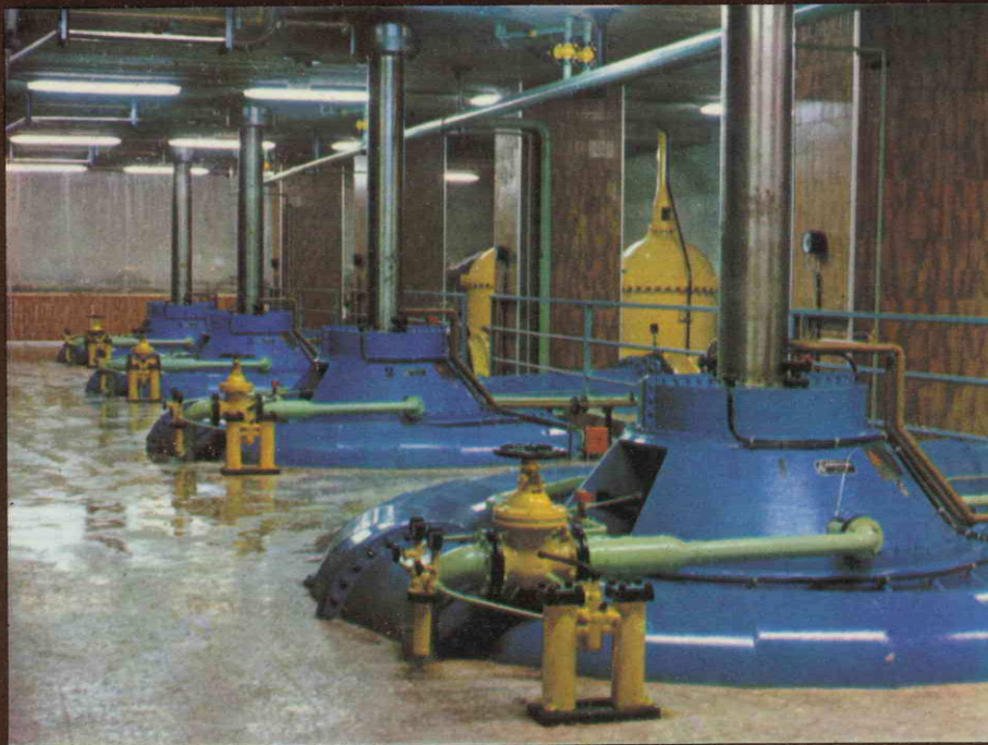
OJÓS PUMPING STATION
