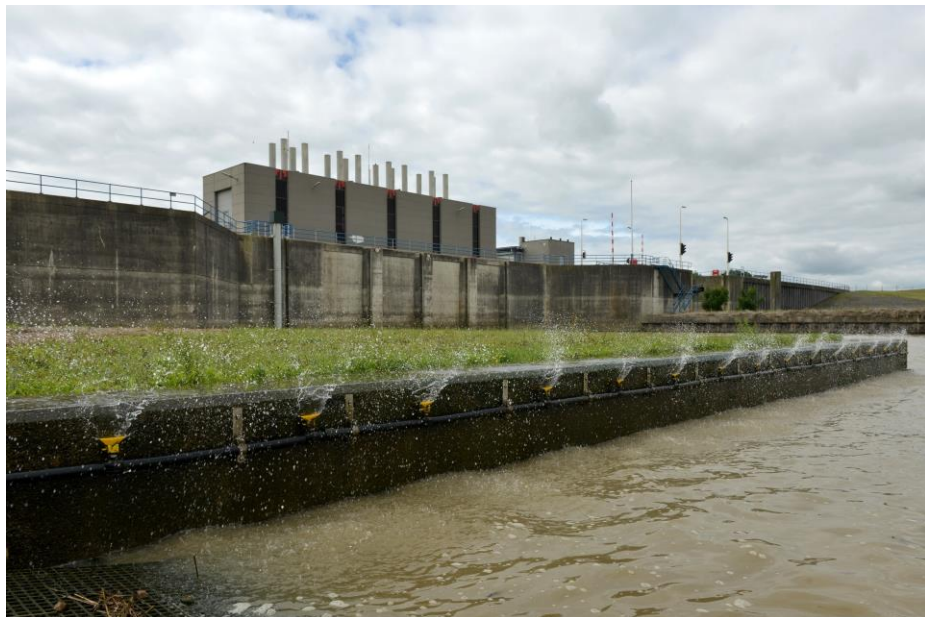
Eel passage at the tidal lock of Nieuwe Statenzijl
